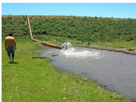
Siphon in operation, water entering the distribution channel
