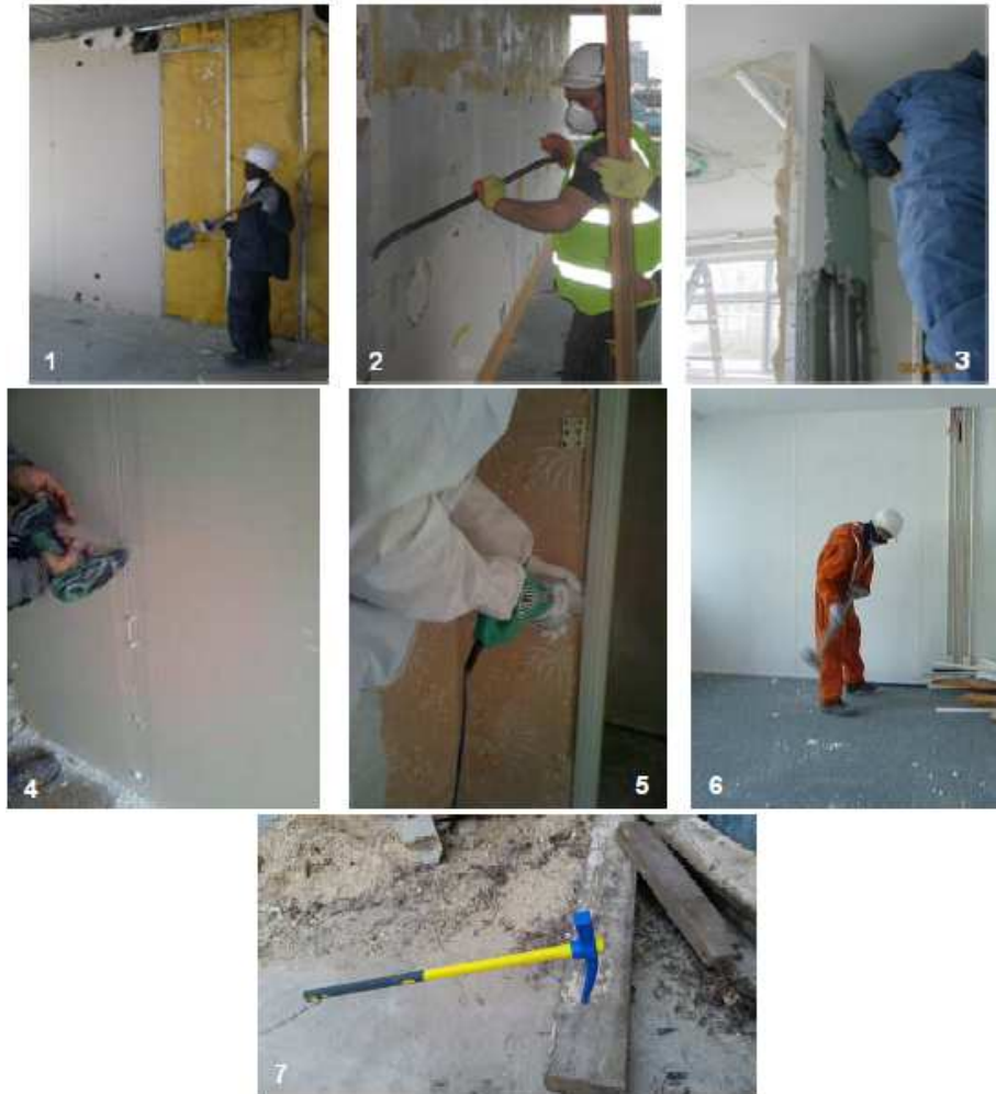
Figure 1. Manual tools generally used to deconstruct gypsum-based systems. Tools used from the picture 1 to the picture 7: shovel, wrecking bar, cutting chisels, automatic screwdriver, saber saw, sledgehammer and pickaxe (Burgy et al. 2015).
