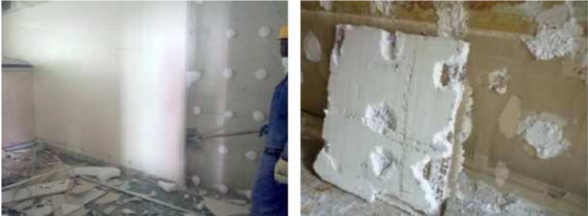
Figure 2. An example of deconstructing sandwich structures glued together using a shovel for leverage, in this case plasterboard and expanded polystyrene attached to a bearing wall. The materials rather than the glue line breaks rendering contaminations in the waste fraction. It is labour intensive and cause crumbling of the material (Burgy et al. 2015).
